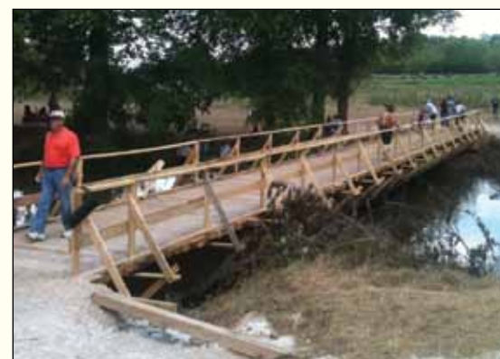
A sturdy wooden bridge was among the major projects financed by the Wilson's Creek Battlefield Foundation leading up to the re-enactment. The structure will remain on the private property.
